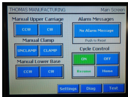
HMI Touchscreen with Automatic and Manual Controls
